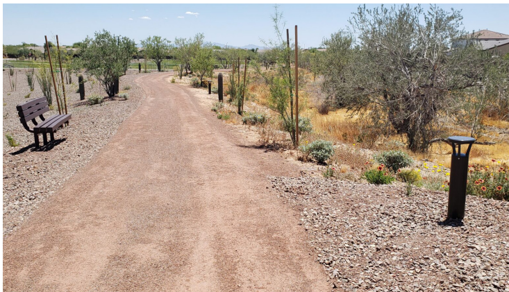
Example of solar-powered lighting bollards along a trail / park
